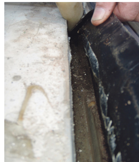
Gootschade, afgebroken rand.
